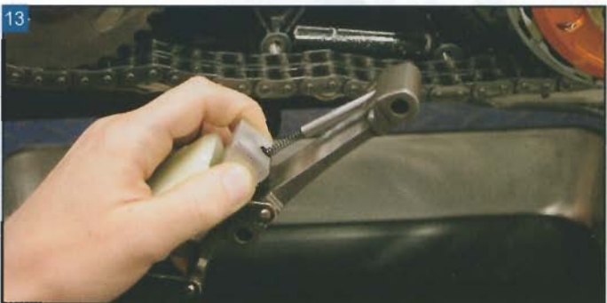
13 Slip the wedge block into the hydraulic chain tensioner assembly as shown.
